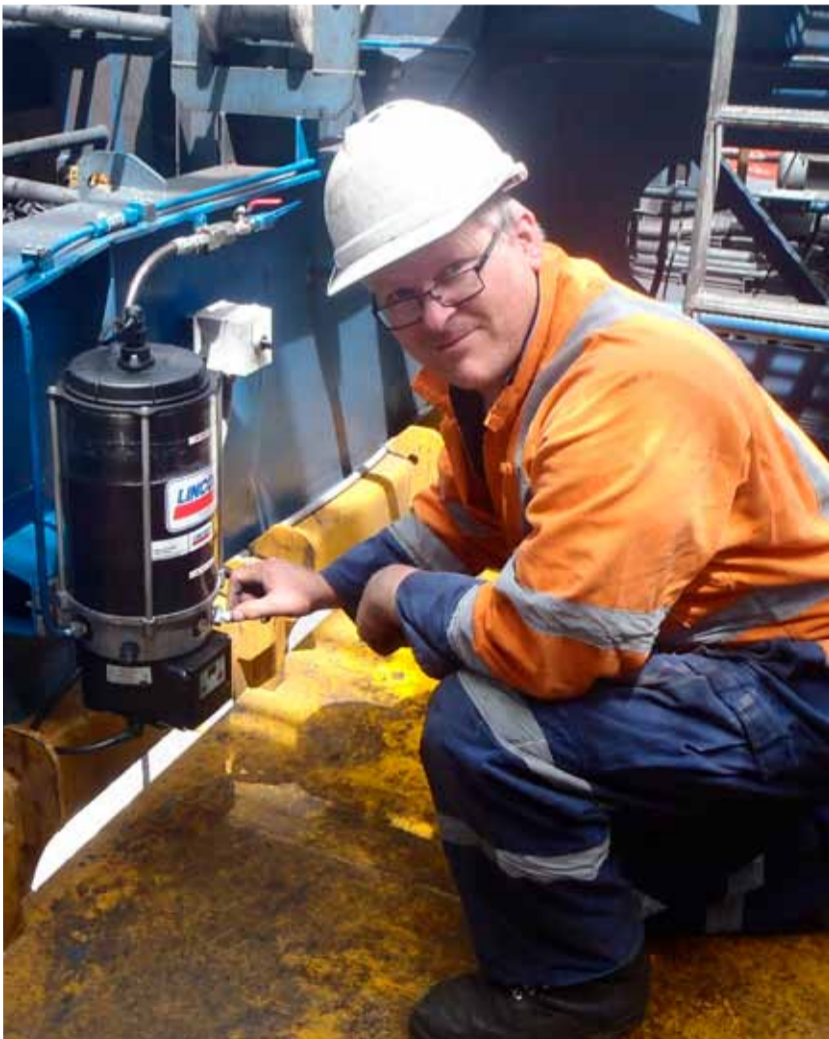
The project's Leading Hand and Field Service Engineer Greg Donald completes the final installation of the trolley auto lube system on one of the Ports of Auckland ship to shore cranes.
