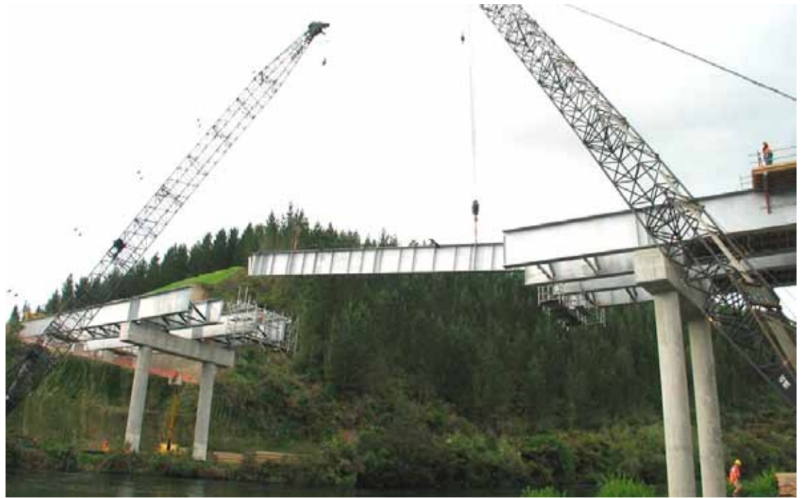
The new Atiamuri Bridge as one of the stringers (bridge beams) is put in place by crane. Images supplied courtesy of NZTA.
